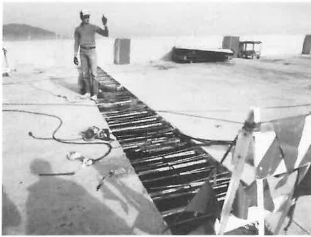
Fig. 11 — Closure strips in slabs were opened up for inspection and repair of floor slab strands.
