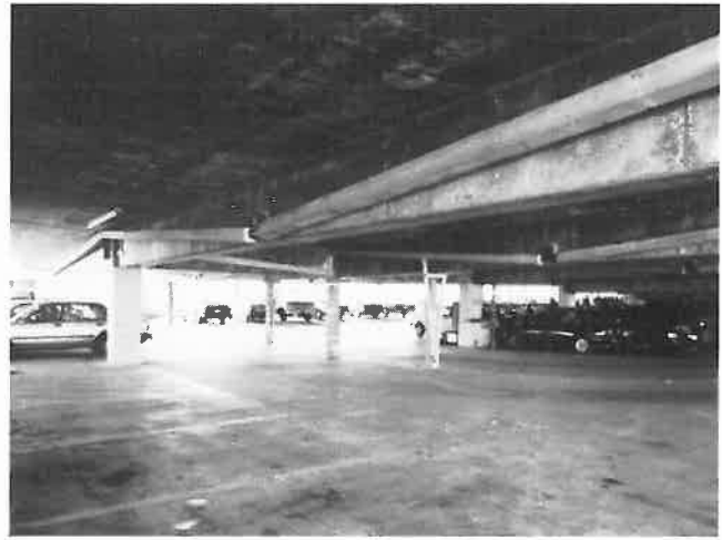
Fig. 12 — After stressing operations, the shoring was removed and the garage was returned to full operation.
